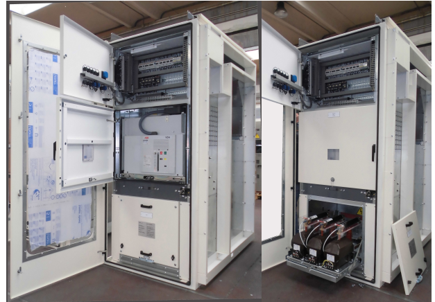
INDONESIA - Centrale geotermica Geothermal power plant
